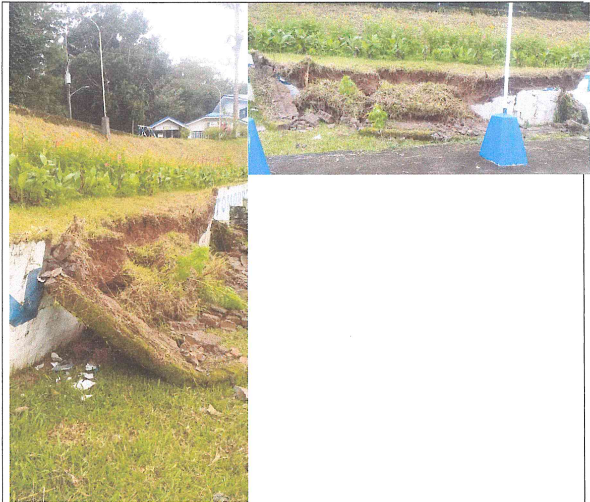
Retaining wall at the Land bridge due for repair
