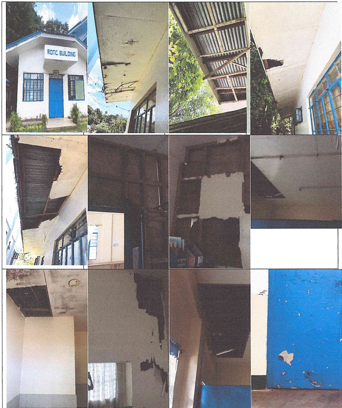
Damages in the ROTC building that need immediate repair
