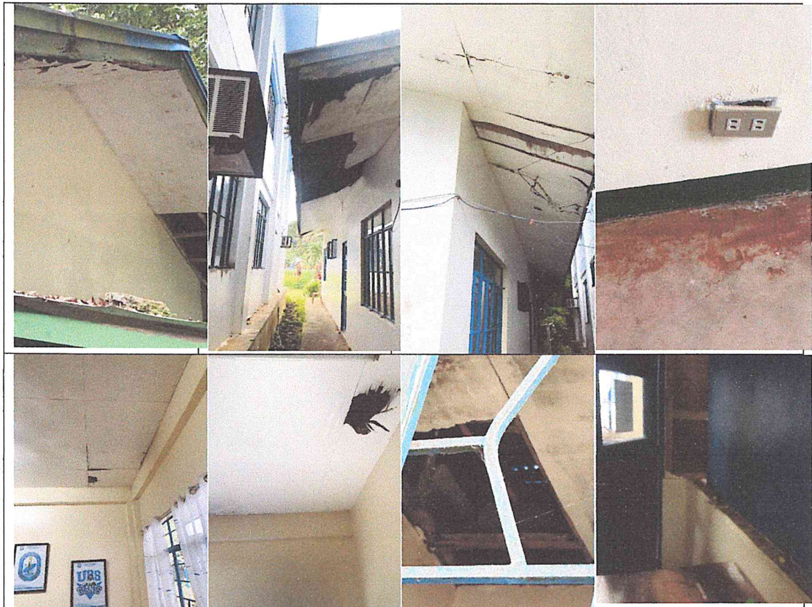
Damages in the ROTC building that need immediate repair
